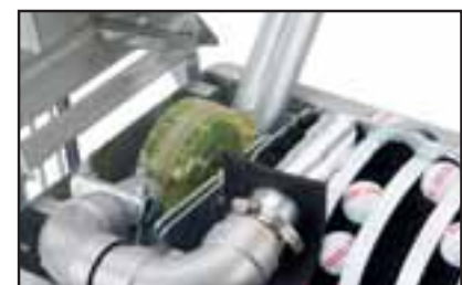
After washing the composite loader wheel pushes the balls into the feeder pipe.
